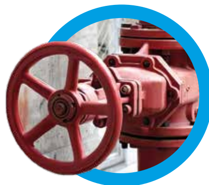
Installation de gaz Gas transportation
