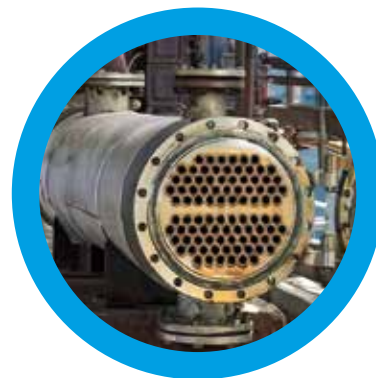
Chaudière Boiler tubes
